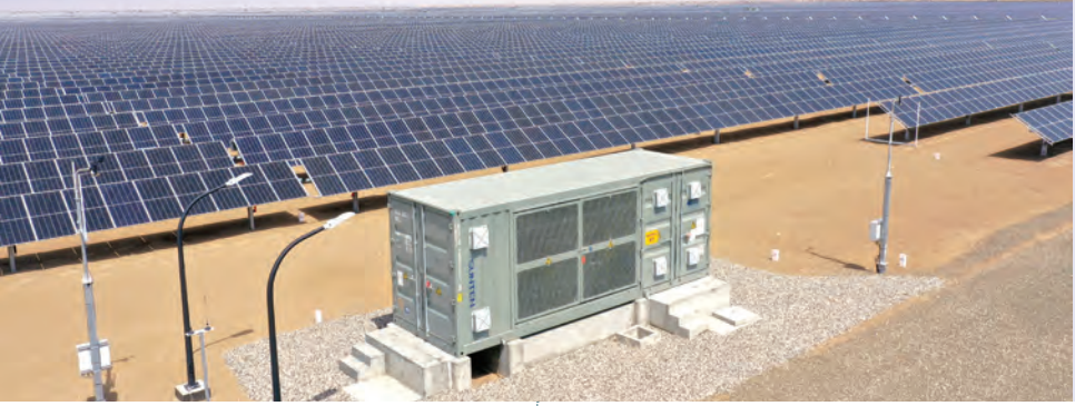
The biggest initiative currently in Solar Wadi’s project pipeline is a 93 MW solar PV plant under development at Suhar Industrial City.
