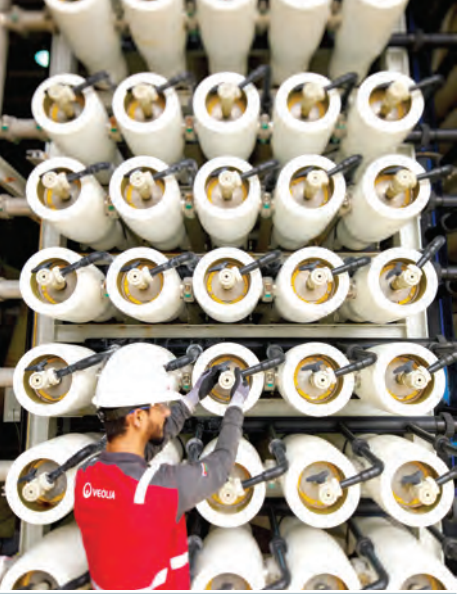
The facility showcases what’s possible when water infrastructure is designed with sustainability at its core.
