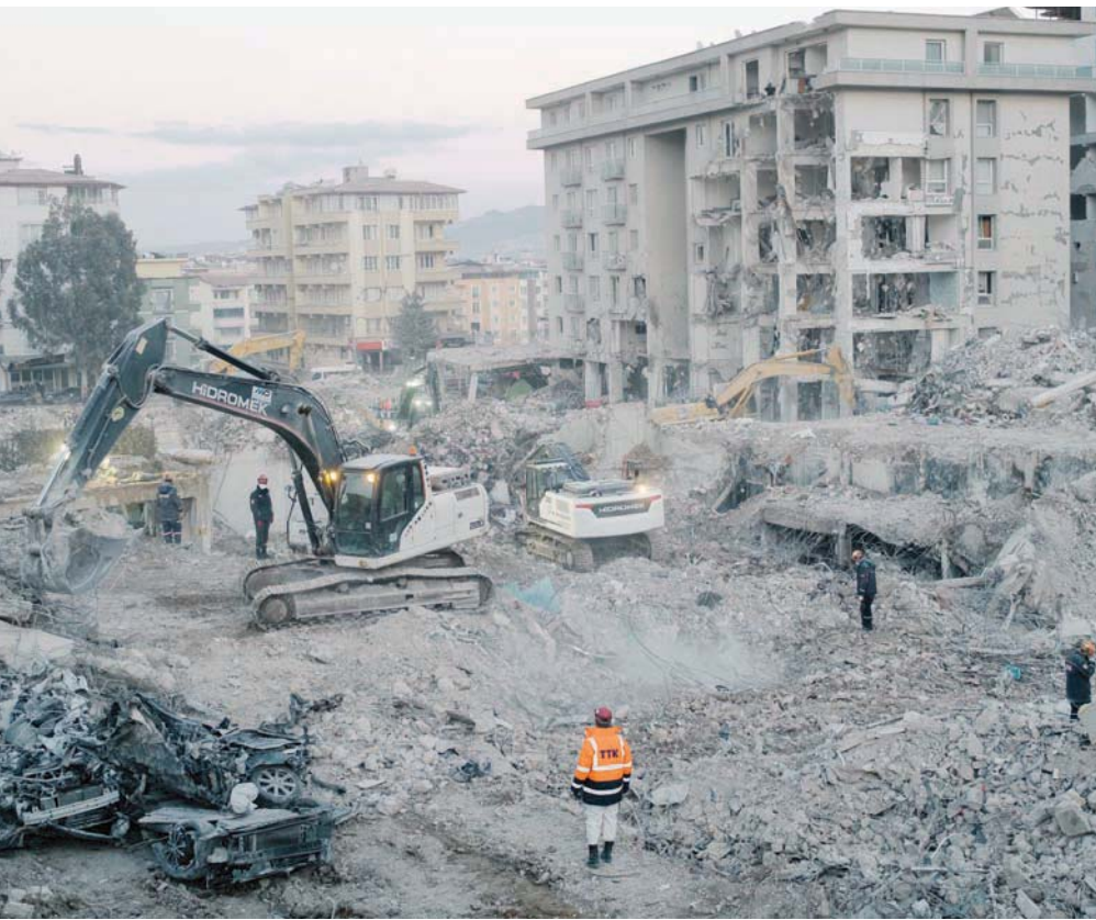
Rescuers at the Renaissance Residence, the site of one of the deadliest building collapses in the 7.8-magnitude earthquake that hit Türkiye on February 6 killing more than 50,000 people and devastating hundreds of thousands of buildings in Ekinçi.
