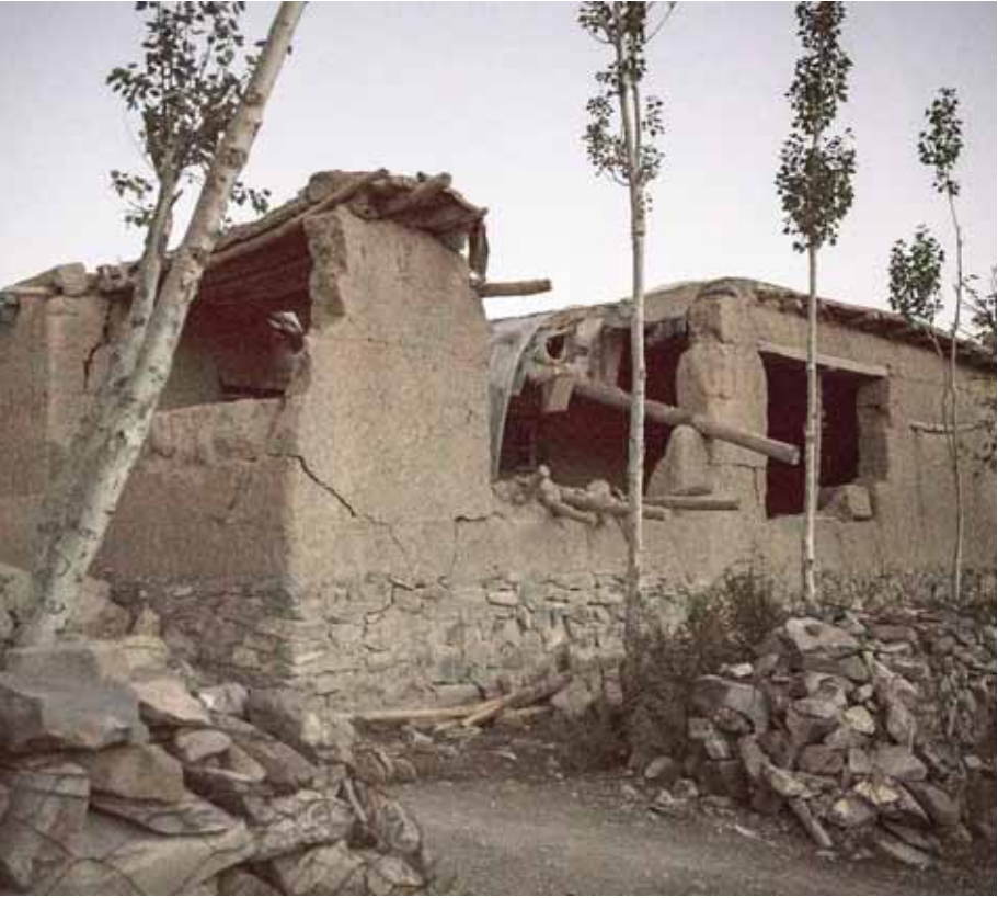
A damaged house in the Geyun district of Paktika Province, Afghanistan.
