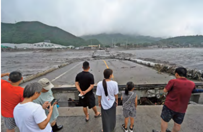
People watch a collapsed bridge on the Dashihe River after heavy rains in Fangshan district in Beijing on Tuesday (AFP)
