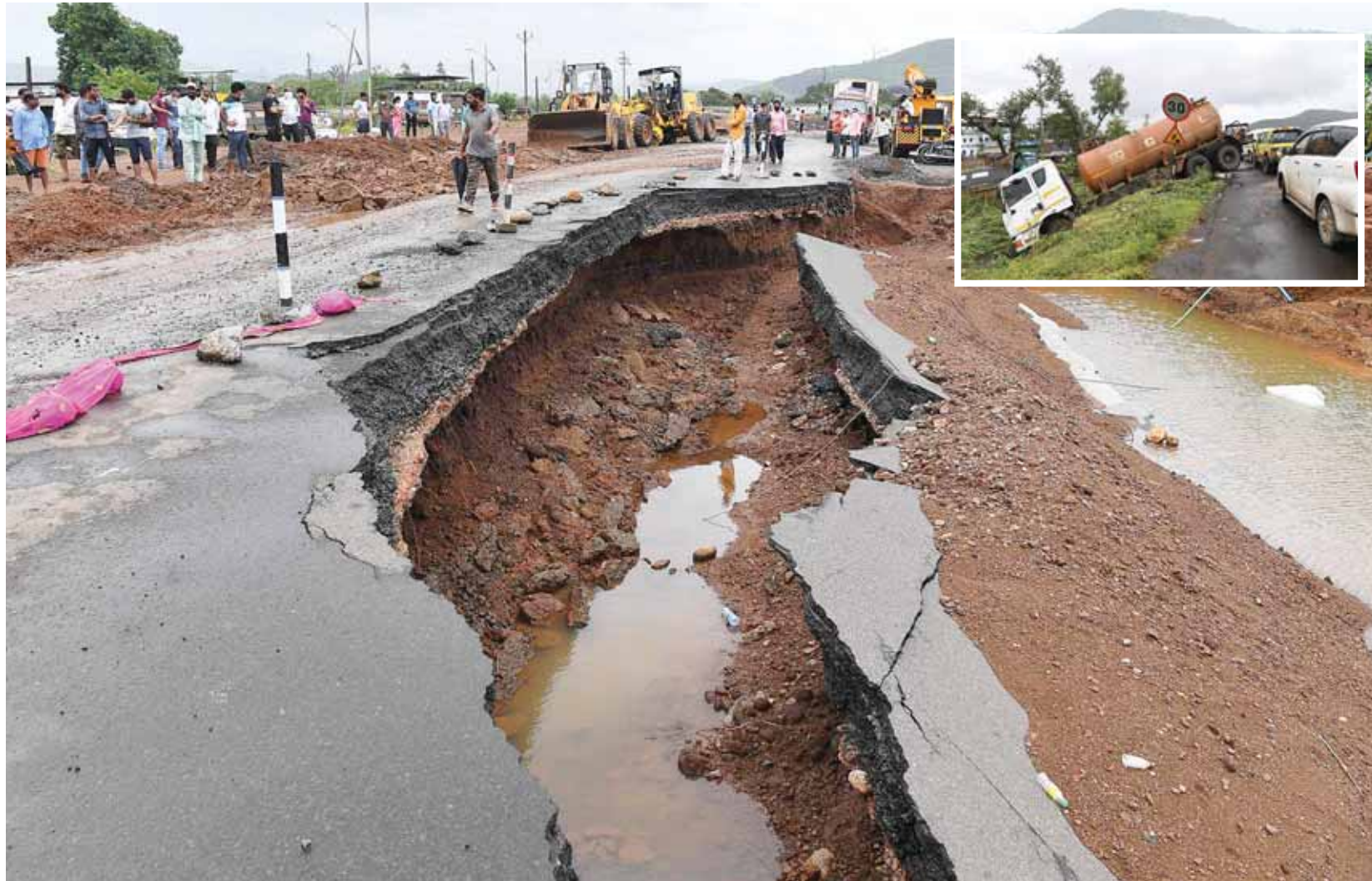
People gather along a section of highway partially washed away from the rain at Mahad with nearly 100,000 others evacuated in Maharashtra. (Inset): A damaged truck lies on the side of a road following a downpour at Mahad. — AFP
