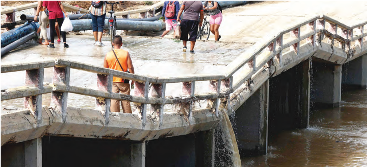
People crosses an affected bridge days after the passage of hurricane Oscar in Guantánamo, Cuba on October 29. — AFP
