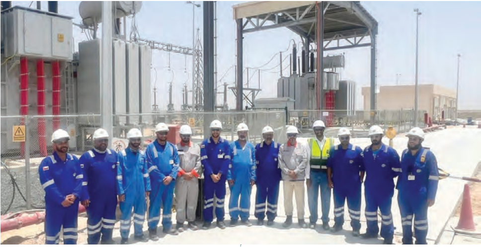
Staff of the OQAE — TotalEnergies JV marking the project's successful energisation.
