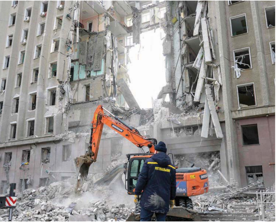
A worker watches an excavator clearing the rubble of a government building hit by Russian rockets in Mykolaiv. — AFP
