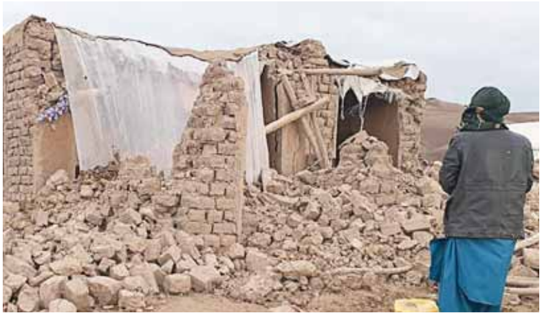
A resident stands near a damaged house at Qadis district in the southern part of Badghis province, after an earthquake hit the region. — AFP
