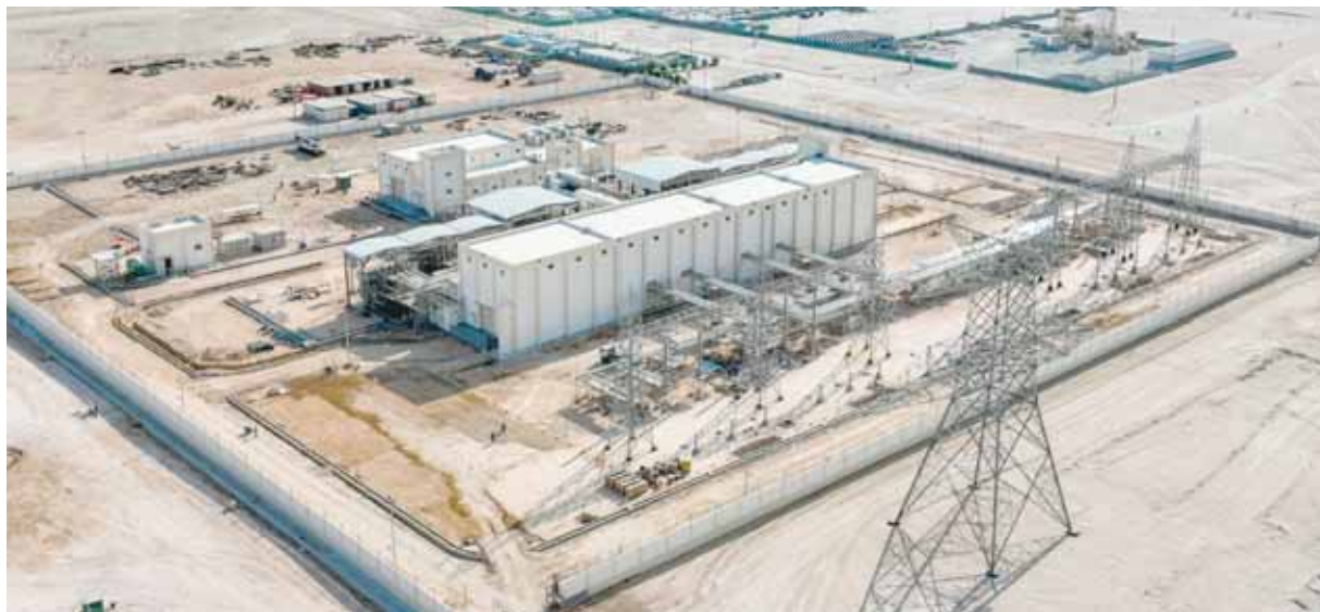
A grid station – one of five built along the route of the Rabt interconnection project.
