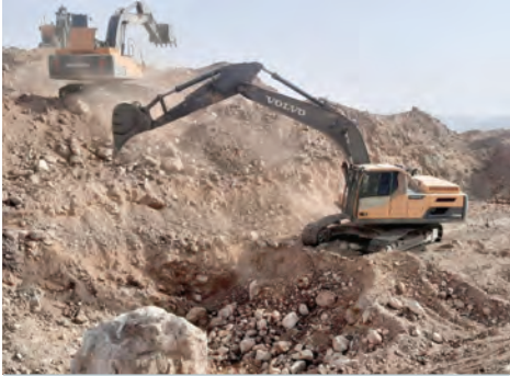
The project includes road safety features such as concrete and metal barriers
