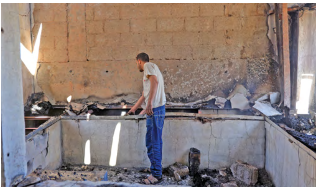
A man inspects a damaged factory following a reported bombardment by the coalition forces in the Houthi-controlled Sanaa, the capital of Yemen, on Tuesday (AFP)
