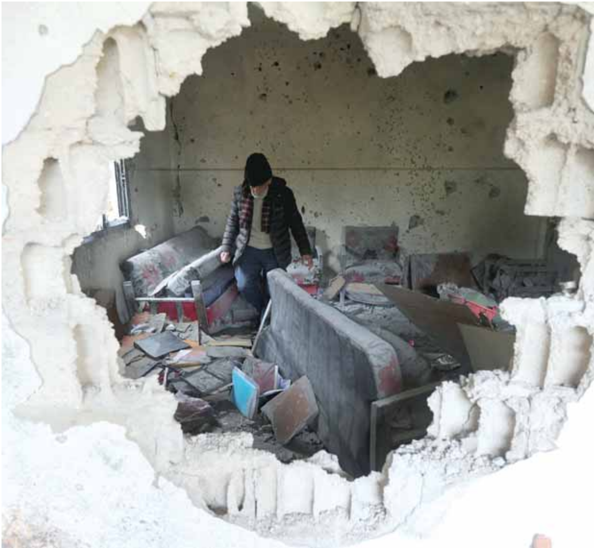
A house that was damaged during Israeli shelling in recent weeks prior to a truce in Mhaibib village, near the Israel-Lebanon border on Tuesday. — Reuters
