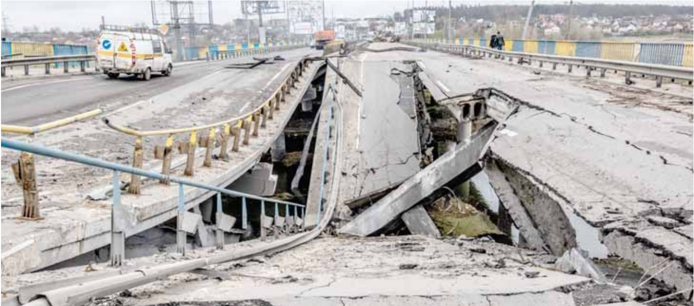
The wreckage of a bombed bridge across the Irpin River in Bucha, Ukraine, near Kyiv.
