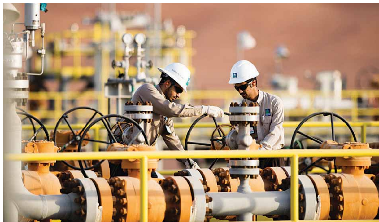
Two men work at an oil pipeline control valves at Saudi Aramco's North Pier Terminal in Ras Tanura, Saudi Arabia. — Reuters
