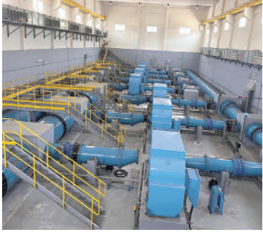
The new pumping station, along with the Al Ghubrah III IWP, will secure the capital city’s potable water needs for the foreseeable future.
