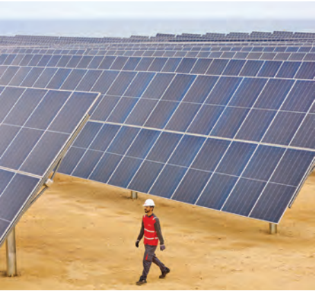
The Sur desalination plant is 100% solar-powered during daylight hours.
