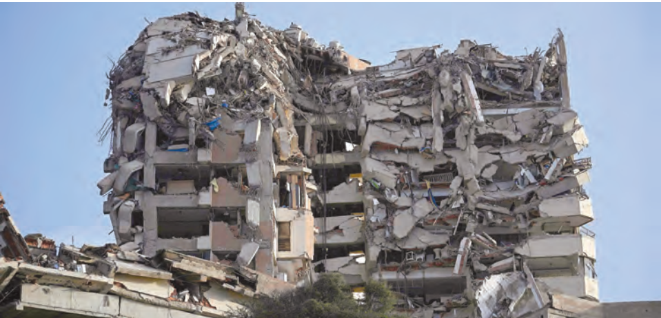
This view shows a heavily damaged multi-storey building with collapsed upper floors in the Playa Verde sector of Catia La Mar. — AFP
