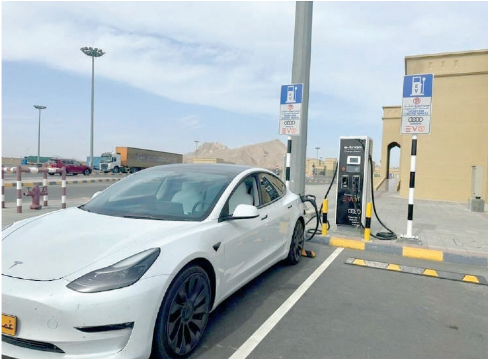
The application will be a unified national platform for charging operators in Oman.
