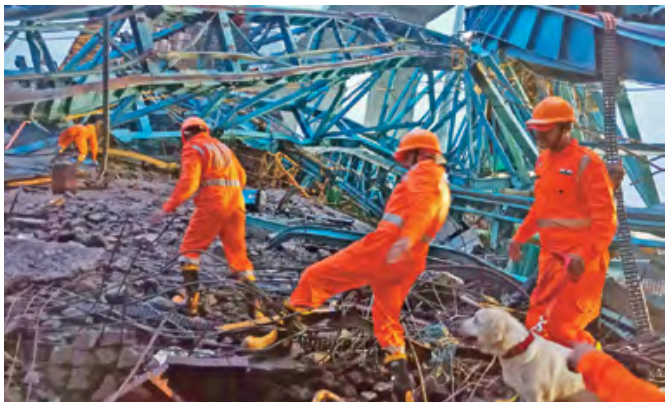
NDRF members inspecting the site of an under construction Samruddhi Expressway where a crane collapsed in Maharashtra on Tuesday (AFP)
