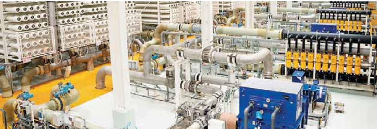
Desalination components at the Barka V plant.
