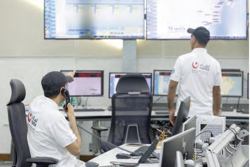
Real-time monitoring of water levels and pumping activity is ongoing through the National Water Monitoring and Control Centre.
