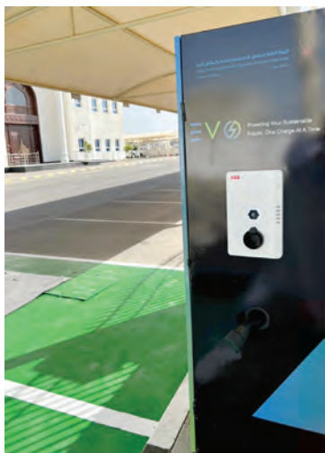
An EV charging station in Muscat, one of many proliferating around the country.
