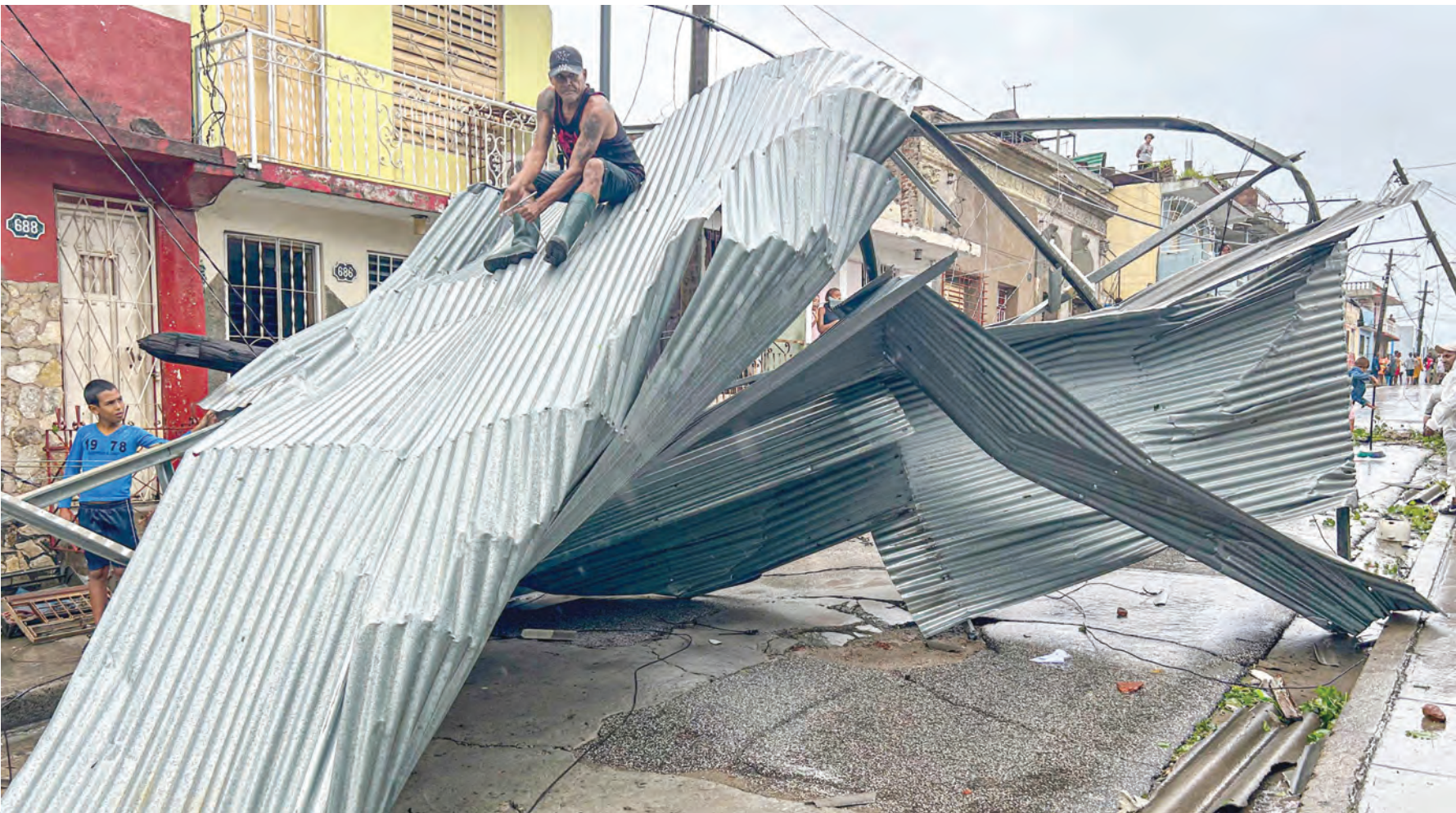
A resident sits on part of the roof of his house, damaged by Hurricane Melissa, in Santiago de Cuba on Wednesday. — AFP
