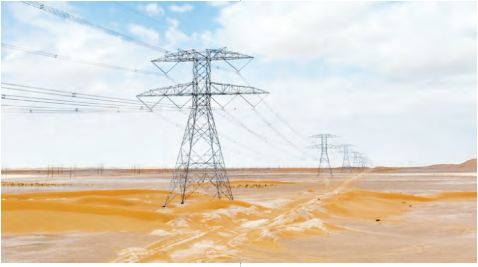
A large portfolio of solar PV and wind farms are planned to be integrated into the national grid over the next five years.
