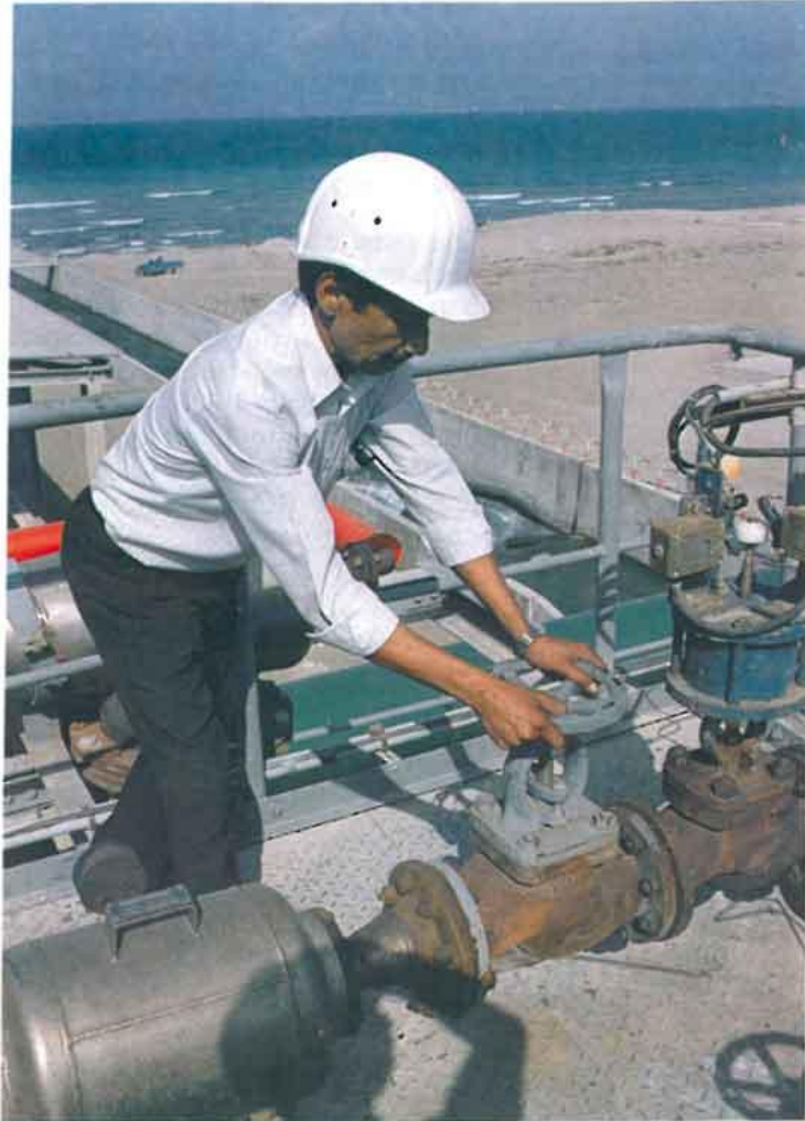
Fresh water for the Capital area — Al Ghubra desalination plant
