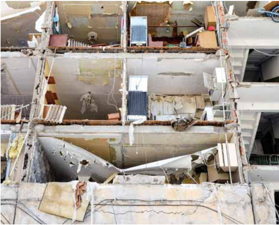
A view of an apartment building heavily damaged after a Russian rocket exploded just outside it in Kharkiv amid the ongoing Russia's war with Ukraine. — AFP
