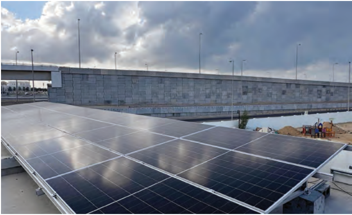
The solar system is expected to generate approximately 336 MWh of clean electricity annually.
