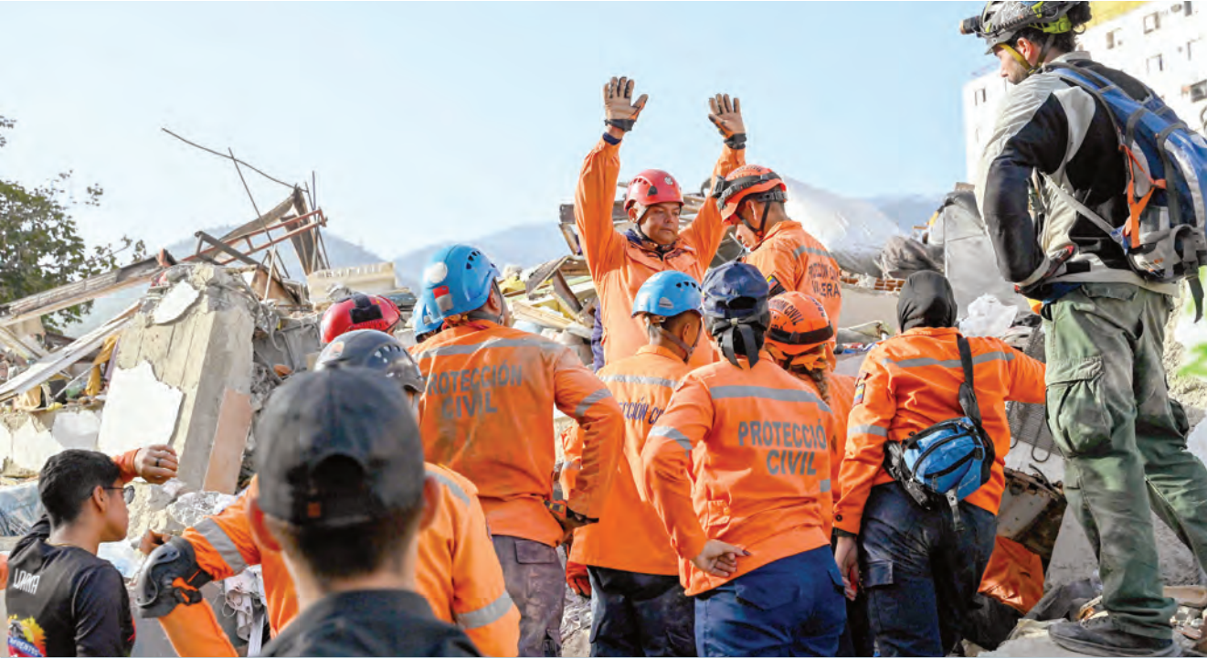
Venezuelan Civil Protection members work at the site of a collapsed building in Caraballeda, La Guaira state. — AFP
