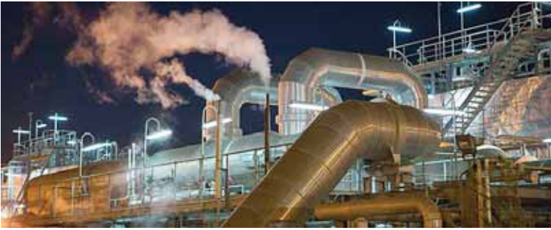
Barka Water and Power confirmed that it met the early power conditions and notified PWP of the plant's readiness for full dispatch capacity of 412 MW.
