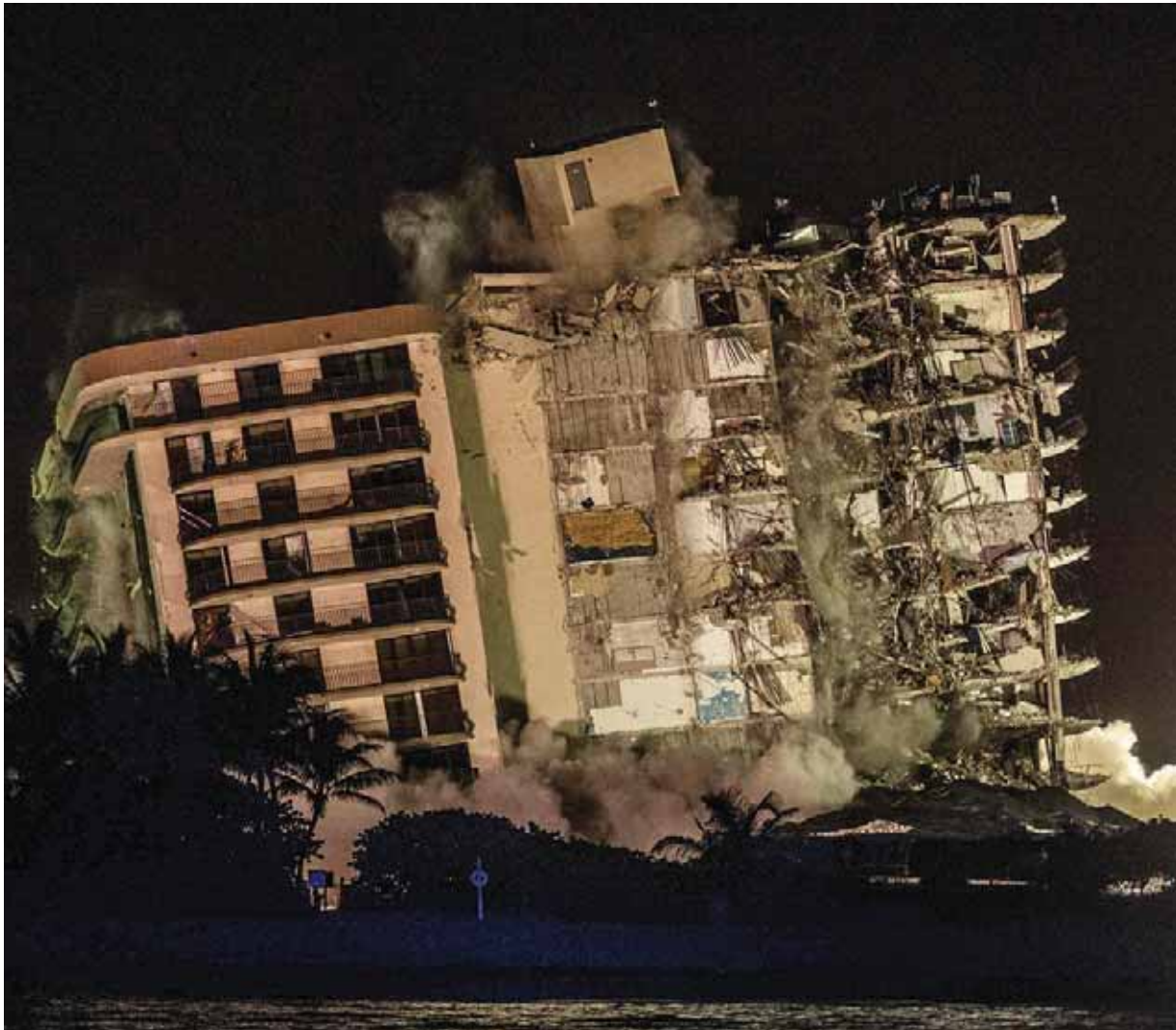
The rest of the Champlain South tower is demolished with a controlled explosion in Surfside. – AFP
