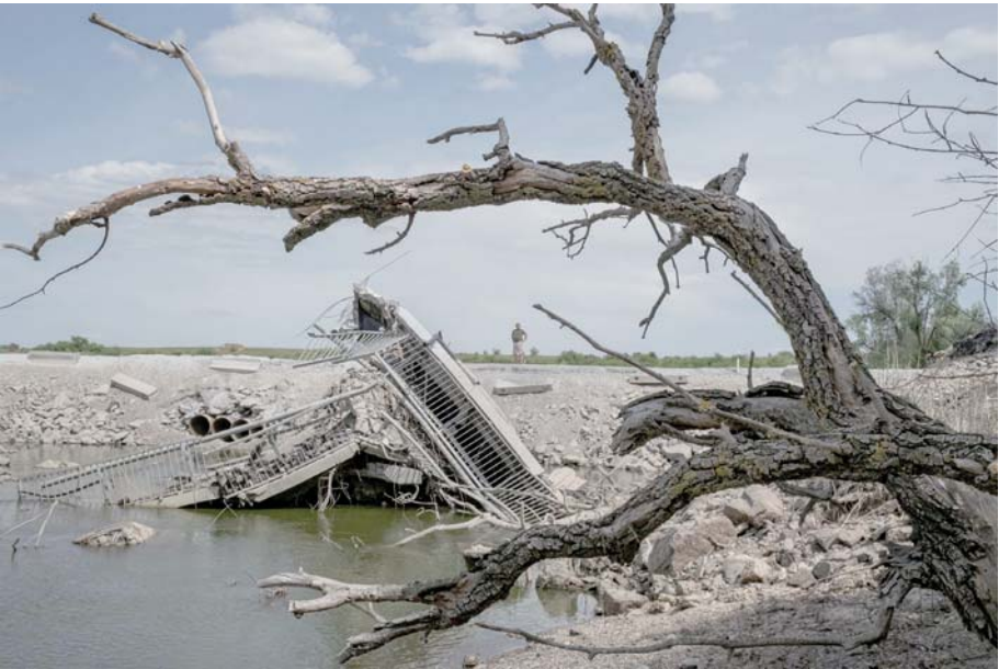
A bridge that collapsed into the water in the Kakhovka dam reservoir after the dam was breached, in the Kherson region of Ukraine.
