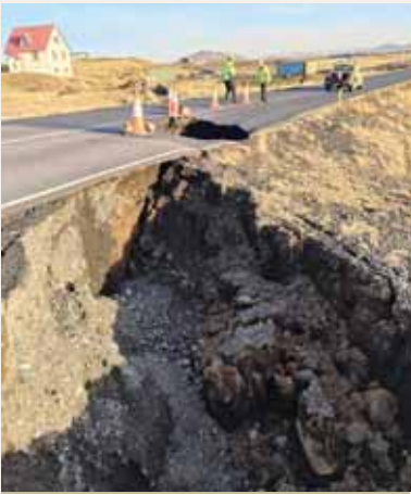
A view of cracks, emerged on a road due to volcanic activity, near Grindavik, Iceland. – Reuters
