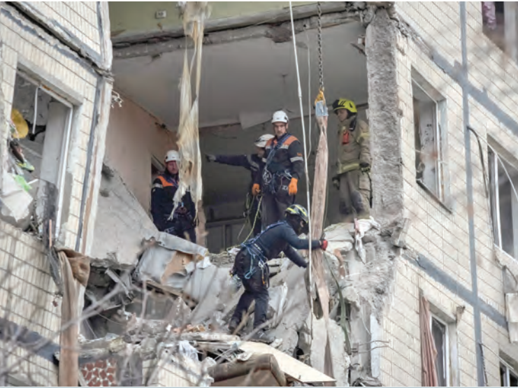
Rescuers work at the site of buildings hit during the Russian drone strike, in Dnipro. — Reuters
