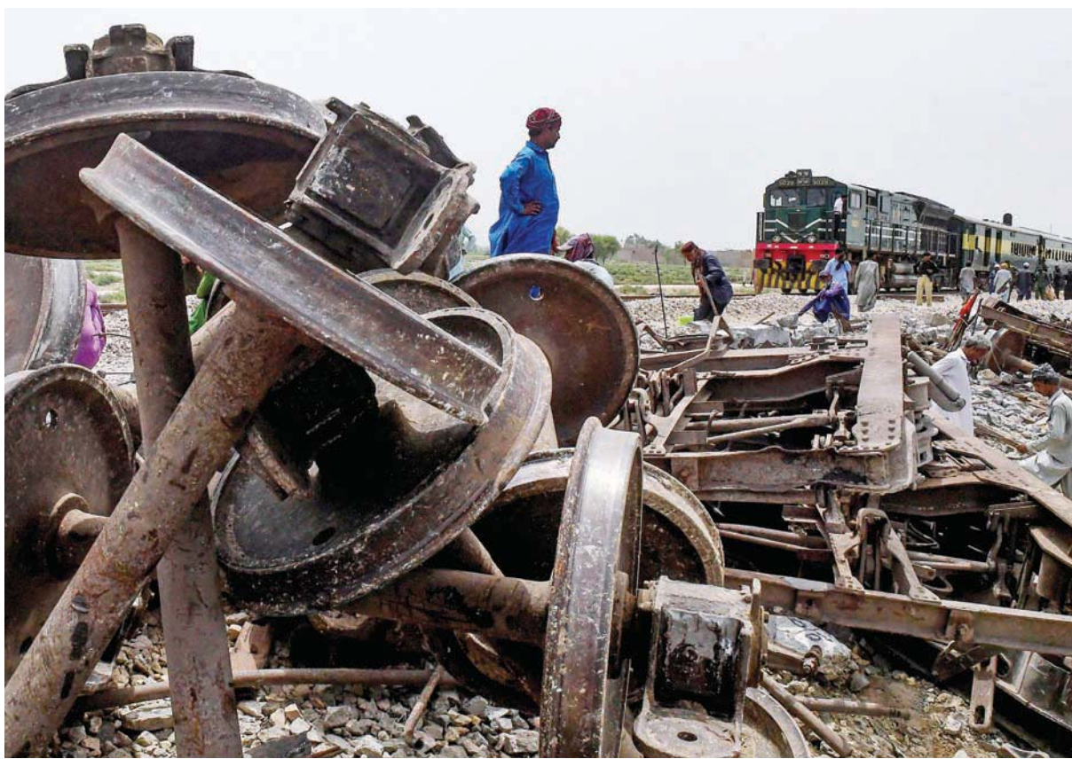
Workers repair a damaged track, a day after the derailment of a passenger train in Nawabshah on Monday. Investigators scoured the wreckage on August 7 of a weekend train derailment that killed at least 34 people, the latest deadly crash to hit Pakistan's antiquated railway network. – AFP
