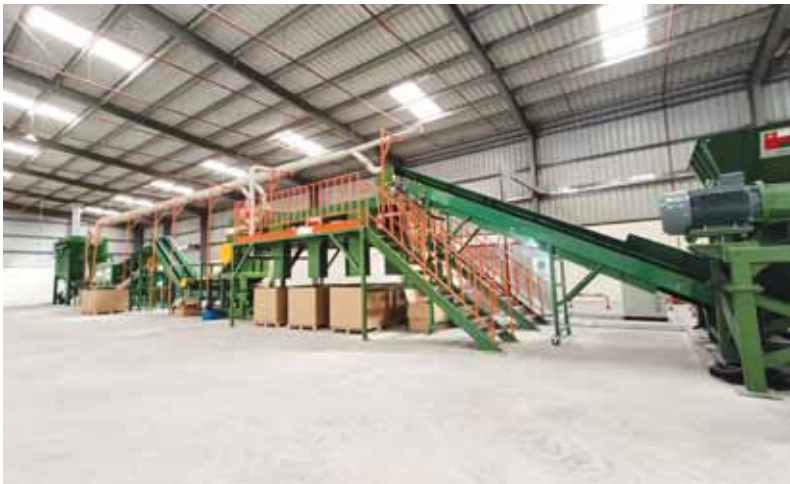
Modern machinery installed at site at the Salalah e-waste recycling hub
