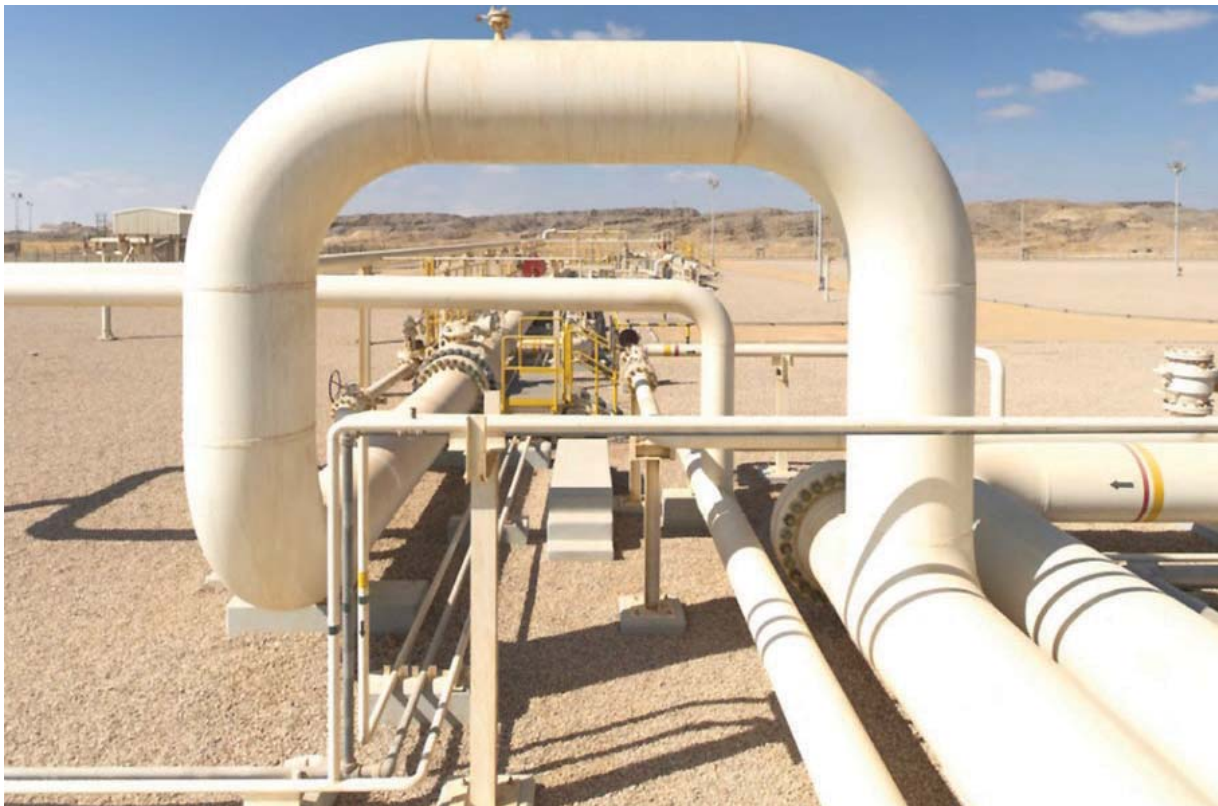
OQGN's oil pipeline is seen in this illustration image.
