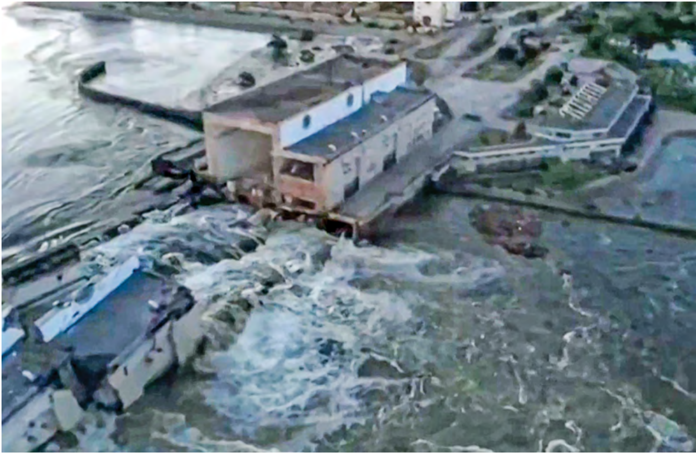
An aerial view of the dam of the Kakhovka Hydroelectric Power Station after it was partially destroyed (AFP)
