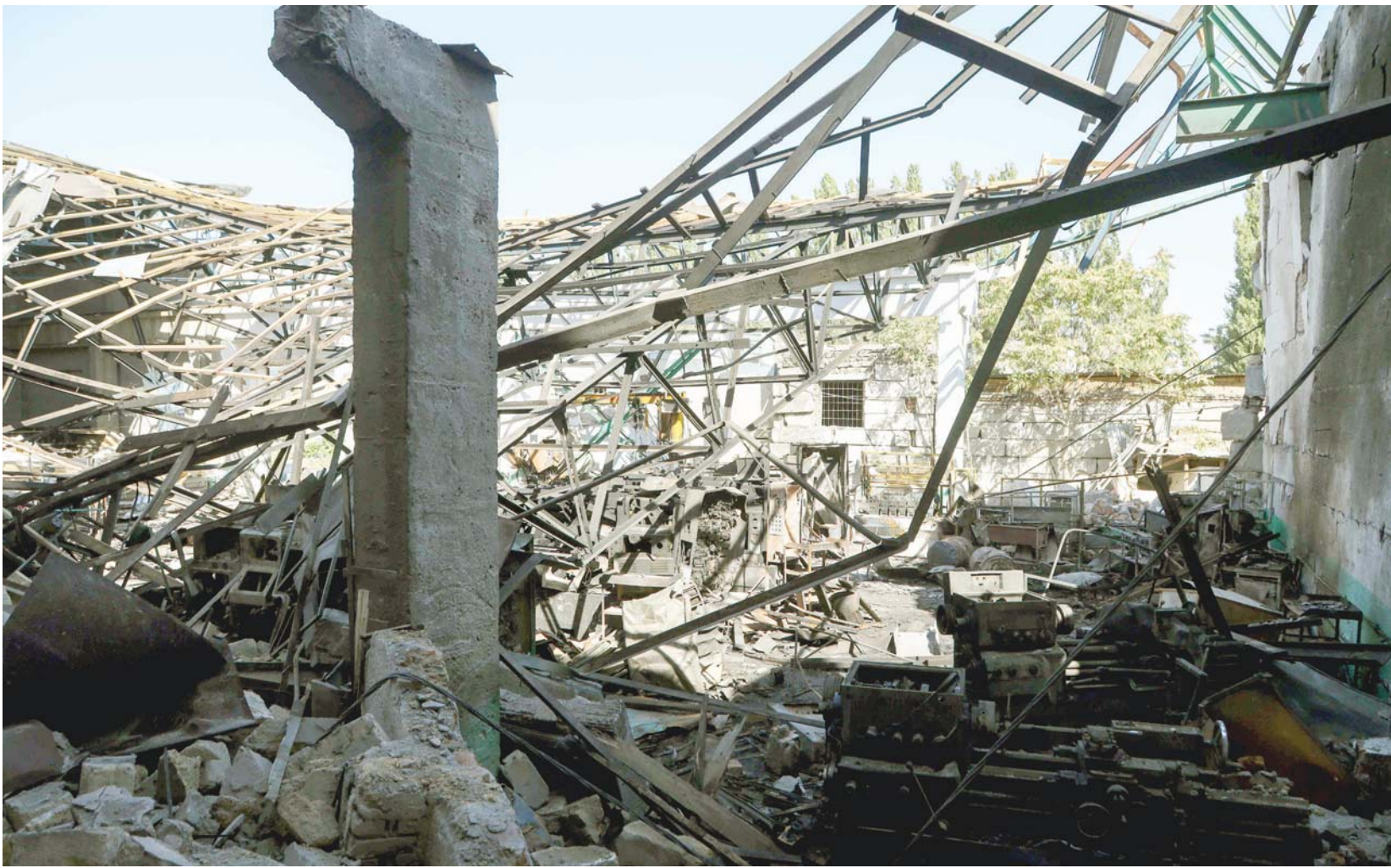
This photograph taken in the Odesa region in southern Ukraine shows an industrial building damaged after a Russian attack. — AFP
