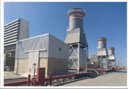
View of Three Gas Turbines
