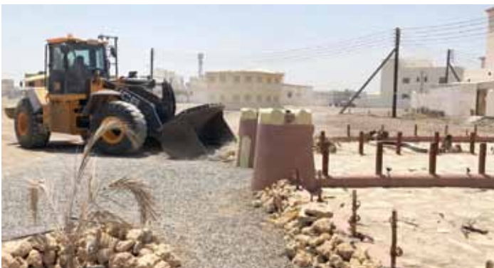
NOT ALLOWED: Encroachments pose a challenge to municipal work and the Muscat Municipality is making all efforts to stop it.
