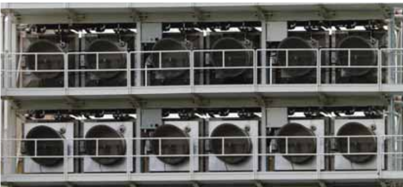
A facility for capturing CO2 from air is placed on the roof of a waste incinerating plant. Image for illustration only. – Reuters
