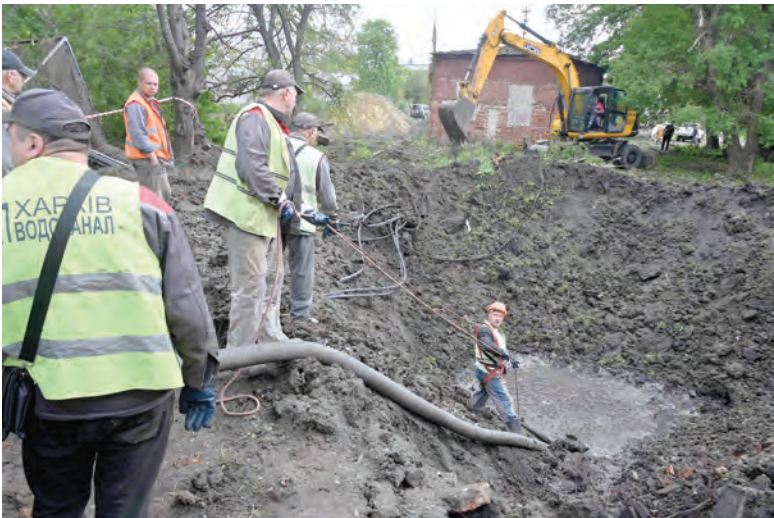
Utility workers operate next to a crater in the courtyard of a hospital in Kharkiv. — AFP
