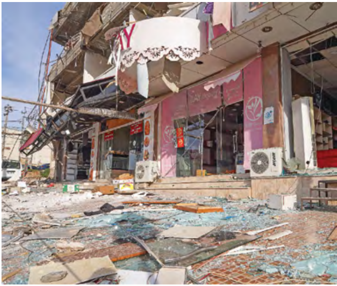
A view of the wreckage left by a gas leak explosion at a student dormitory building in Dohuk on Tuesday (AFP)
