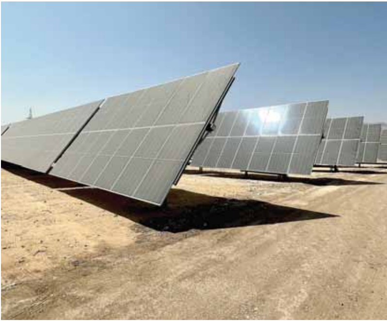
Solar PV farm powering the desalination plant in Sur.
